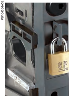
"Disconnected" position locking by padlocks.
