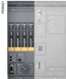
Local information and control
